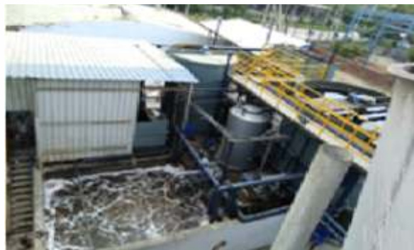
Fig. 39. Effluent treatment plant
